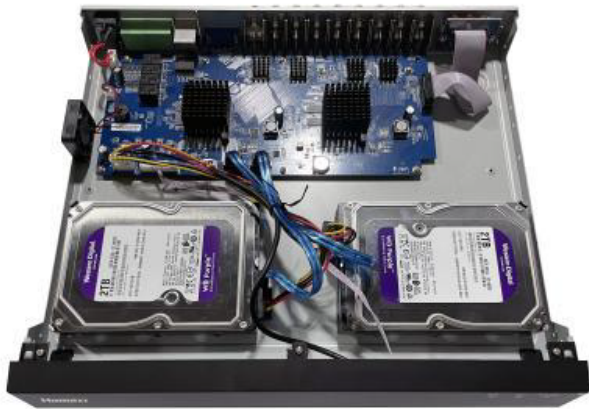
Figure 1-6 Connect the power and data cables
